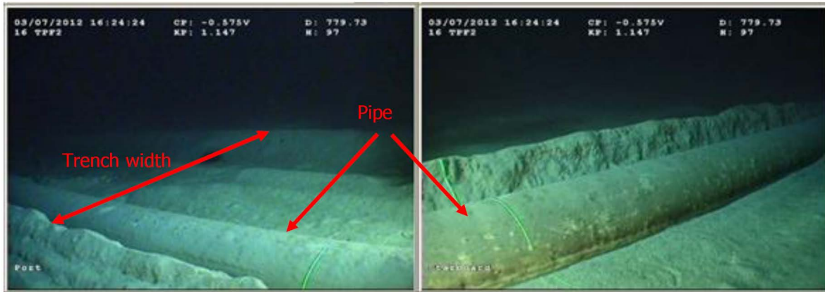
Figure 3—Trench and berms created by the sweeping action of the pipeline at the first lateral buckle
